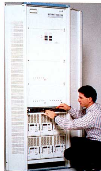
Energy systems. AT&T
