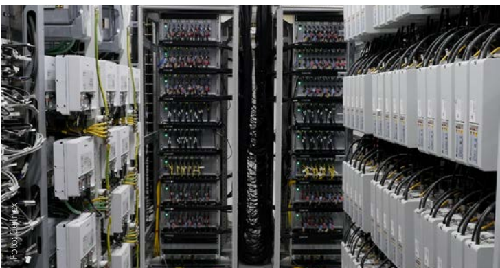
Control Room Wanda Metropolitano
